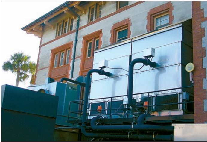
Because of the salt air, water cooled chillers along with a new primary loop were specified for Flagler College.
